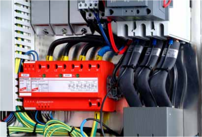
Figure 7.8: Lightning and overvoltage protection system for protecting the AC feed-in system and the control voltage supply
