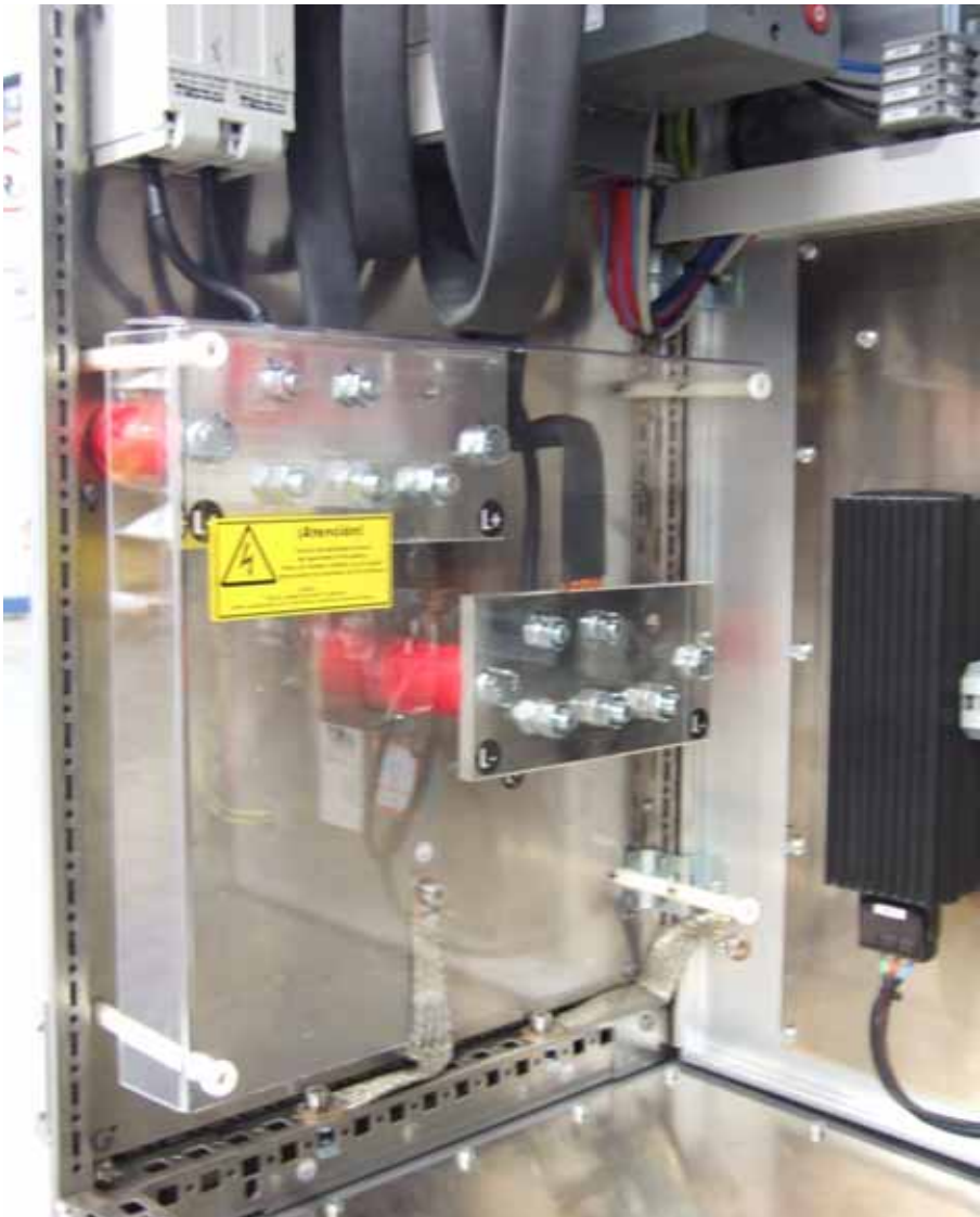
Figure 7.5: View of the DC connection area
